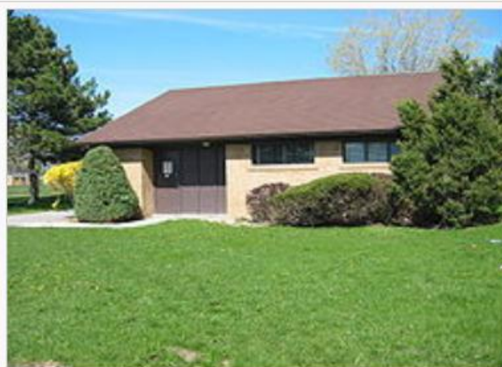
A distribution substation in Scarborough , Ontario disguised as a house, complete with a driveway, front walk and a mown lawn and shrubs in the front yard. A warning notice can be clearly seen on the "front door".
